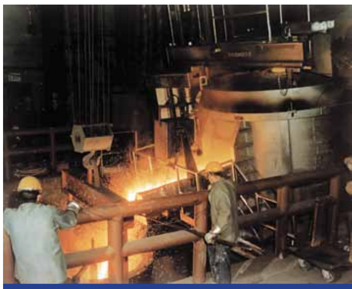
Figure 4. An electric arc furnace represents the latest technology for refining spent PGM catalysts.
